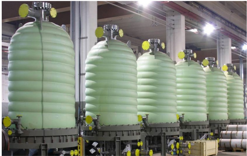
Polysilicon deposition chambers (Ref. Poly Plant Project Inc.)
